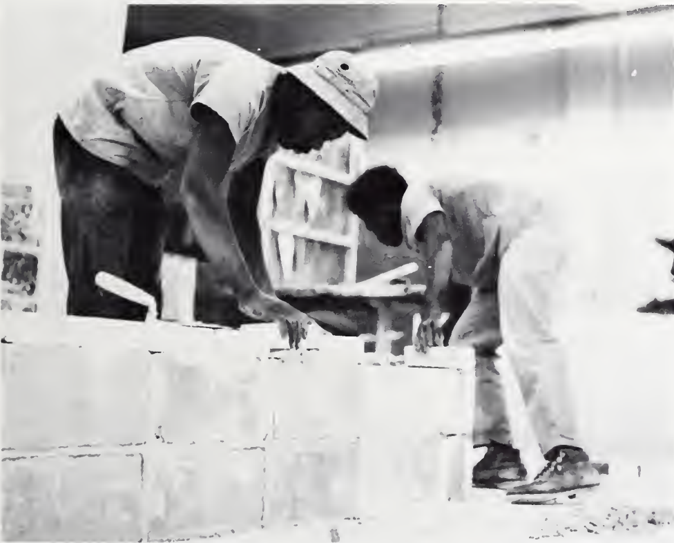
BRUCE PATTERSON and David Gibson lay bricks in Mr. Miessen's Masonry class.
